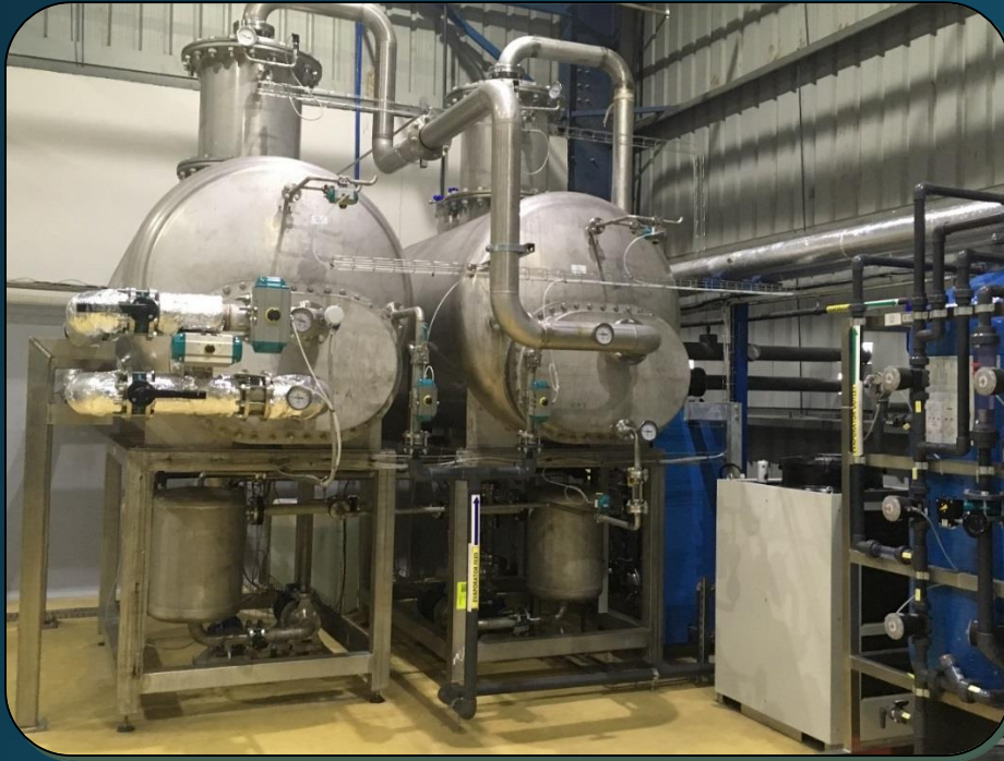
Evaporator Recovery Unit
